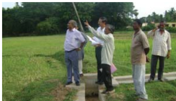
Commissioner, CAD & WM, MOWR, GOI visiting Field Channel work at village Pipili Sasan (Mahanadi-Delta Stage-II)
