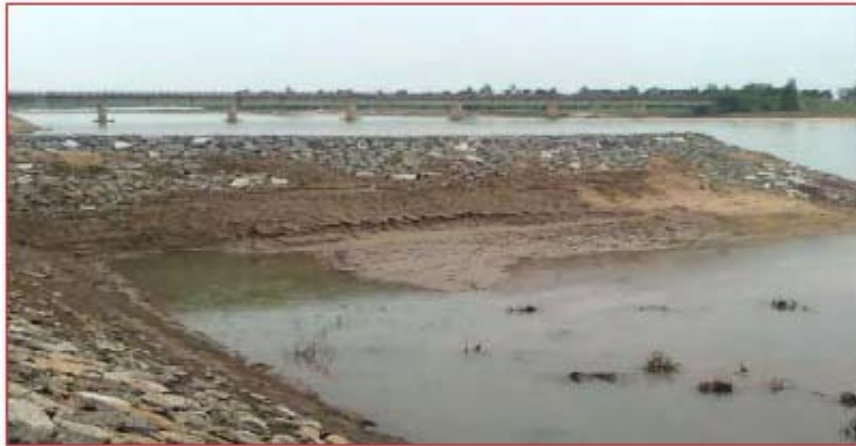
Spur & Slope protection work at RD 17.42 km on River Paika (work Completed under Flood Management Programme)
