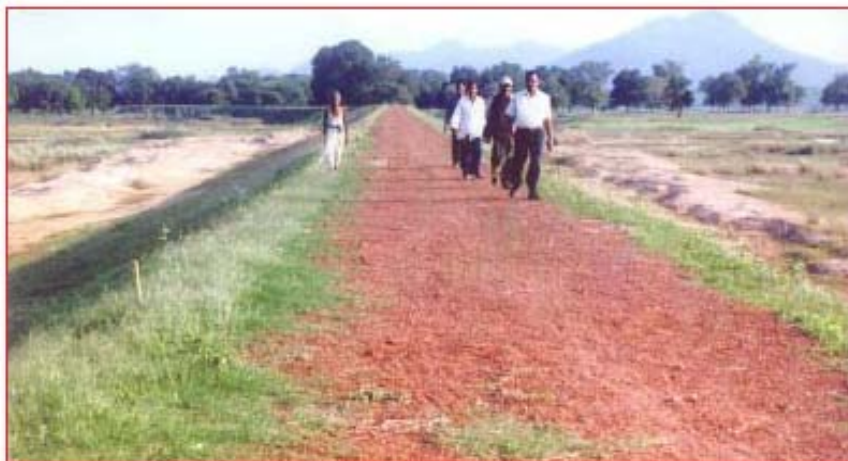
Restoration of marginal flood embankment from Chanipal to Mahurpal on Brahmani Left at village Bhuatal (work in completed under RIDF-XII)
