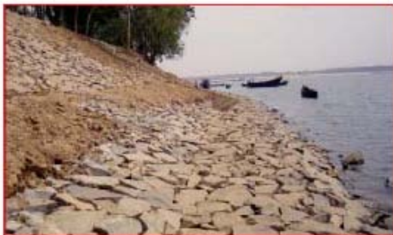
Slope protection work in left bank of river Subarnarekha at Chitimisira (work in progress under FMP)
